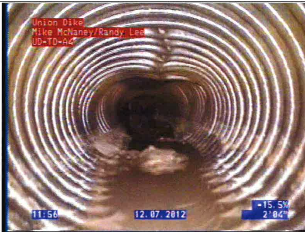
PHOTO 6 - VIEW OF OUTLET A4 - PIPE CRIMPING/BUCKLING
