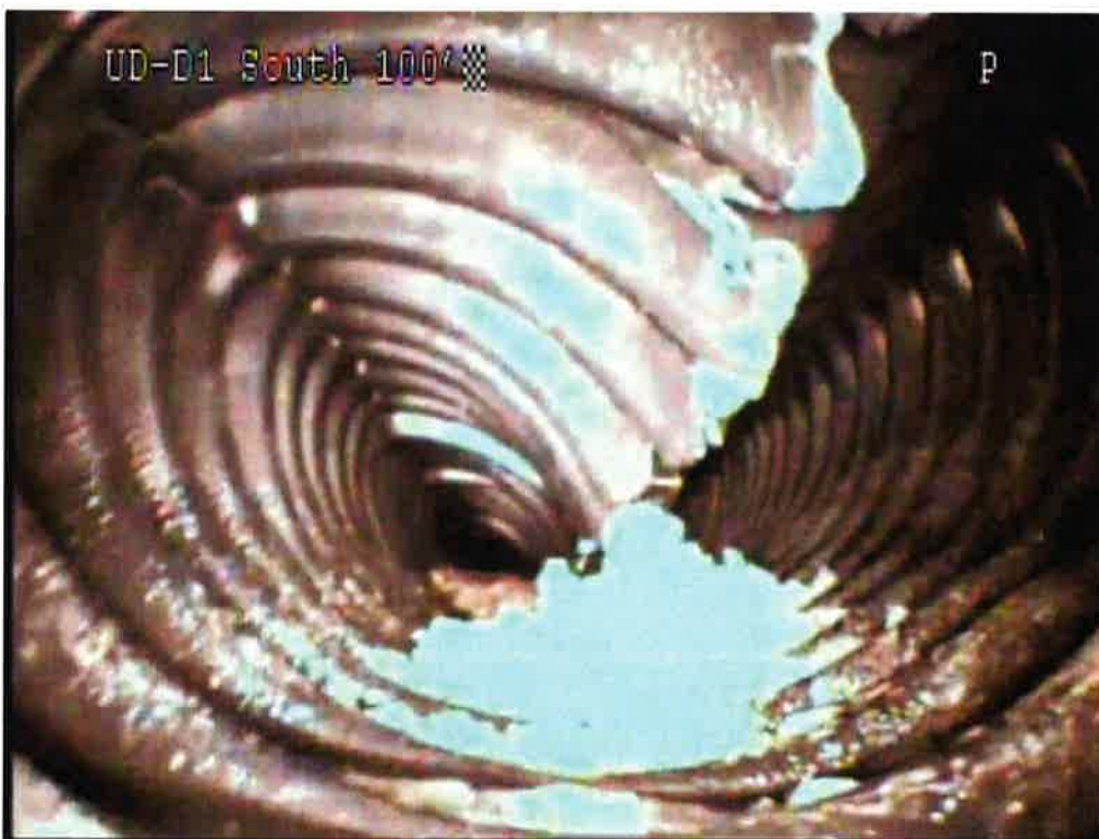
PHOTO 27 - VIEW OF TRENCH DRAIN SOUTHEAST OF OUTLET D1 - PIPE BUCKLED/COLLAPSED
