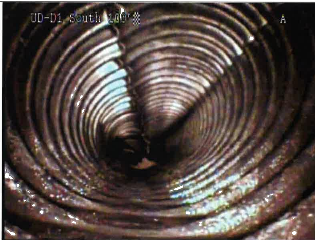
PHOTO 26 - VIEW OF TRENCH DRAIN SOUTHEAST OF OUTLET D1 - PIPE BUCKLED/COLLAPSED
