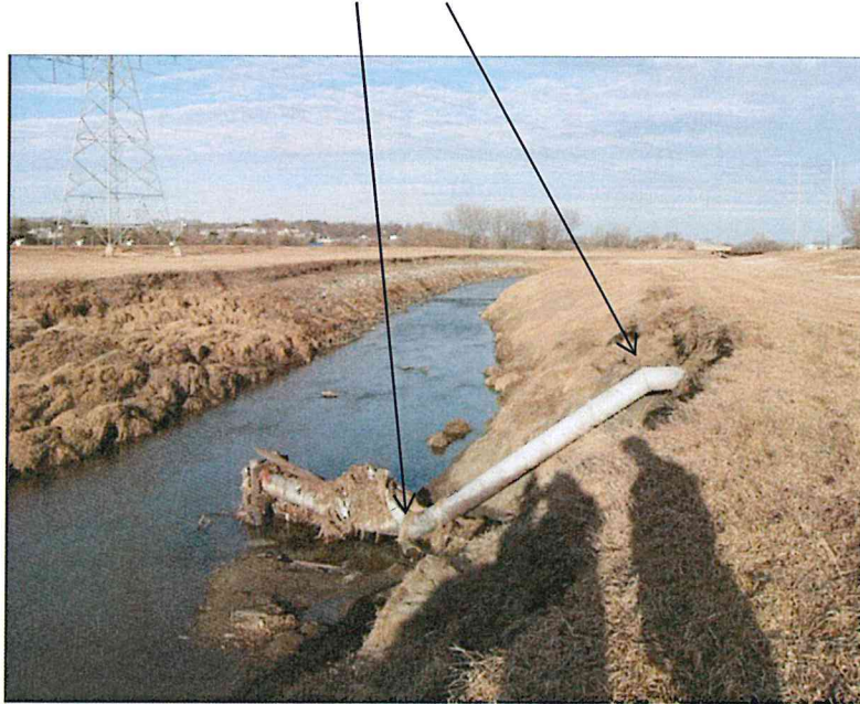
Example of pipe with double breaks
