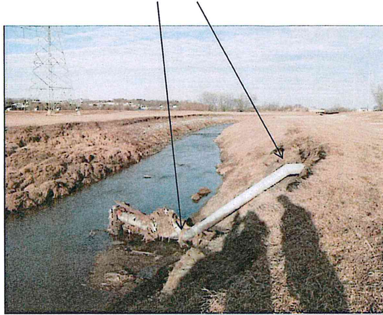
Example of pipe with double breaks
