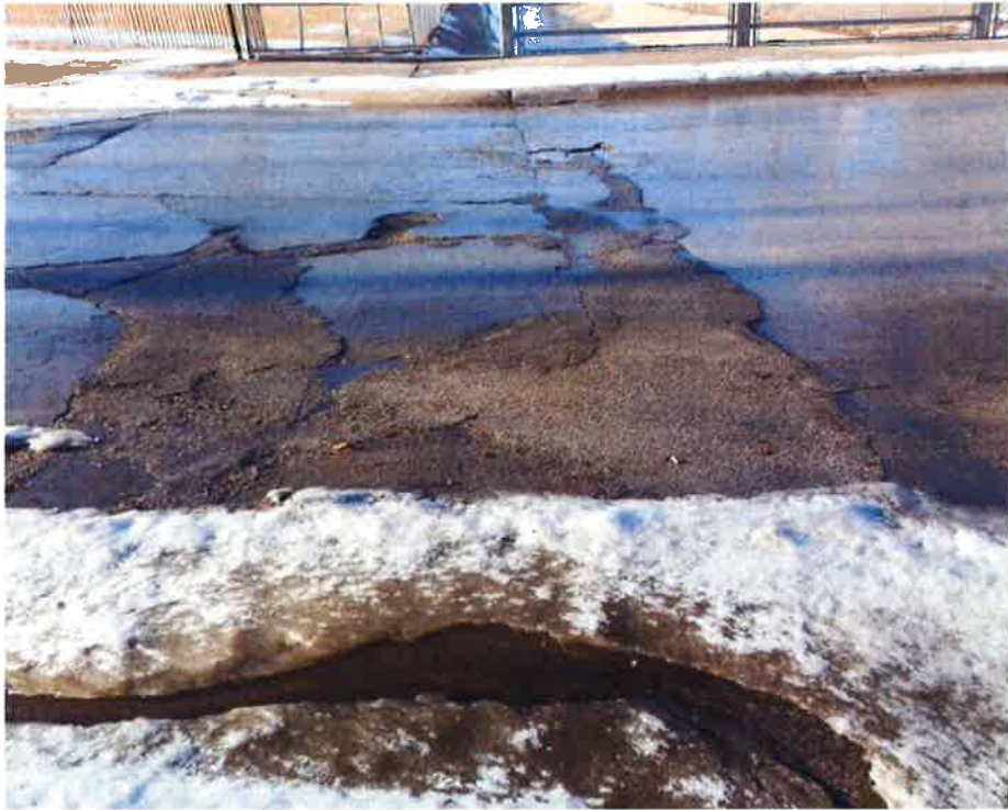
FIGURE 6 – TYPICAL CONCRETE CRACKING AND POTHOLES ON DECK AT A STREET
