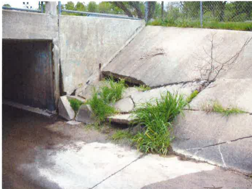
FIGURE 4 – TYPICAL CONCRETE LINER FAILURE UPSTREAM OF C STREET
