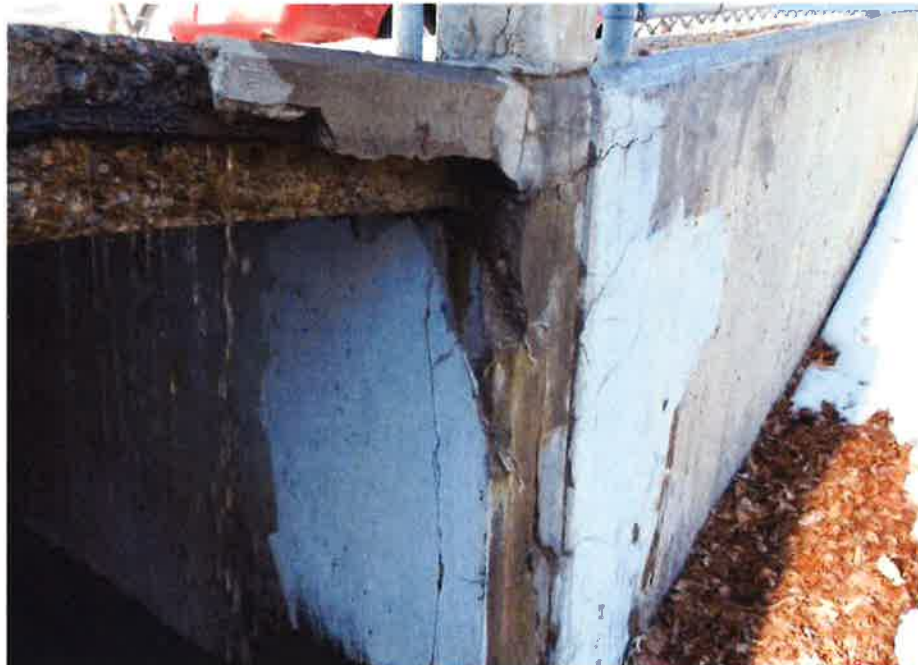
FIGURE 7 – TYPICAL EXPOSED REINFORCING STEEL FROM DELAMINATED CONCRETE AT A STREET
