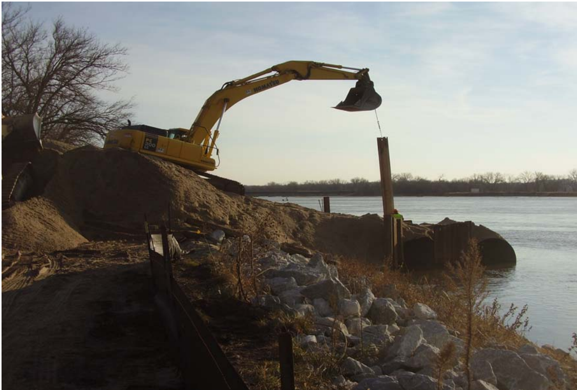
Photo: The Contractor continues to haul sand as well as begin construction of the causeway. Date: November 27, 2007
