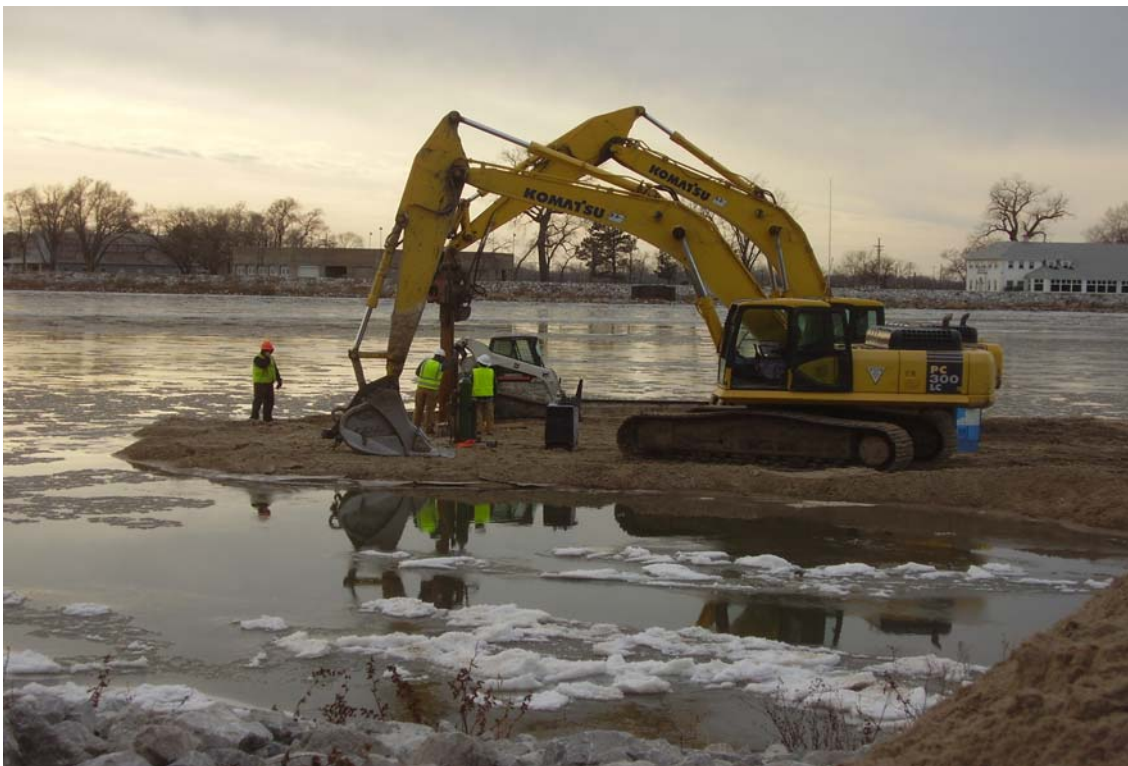
Photo: The Contractor has located piers 7S and 7N and has started construction of the cofferdam. Date: November 30, 2007
