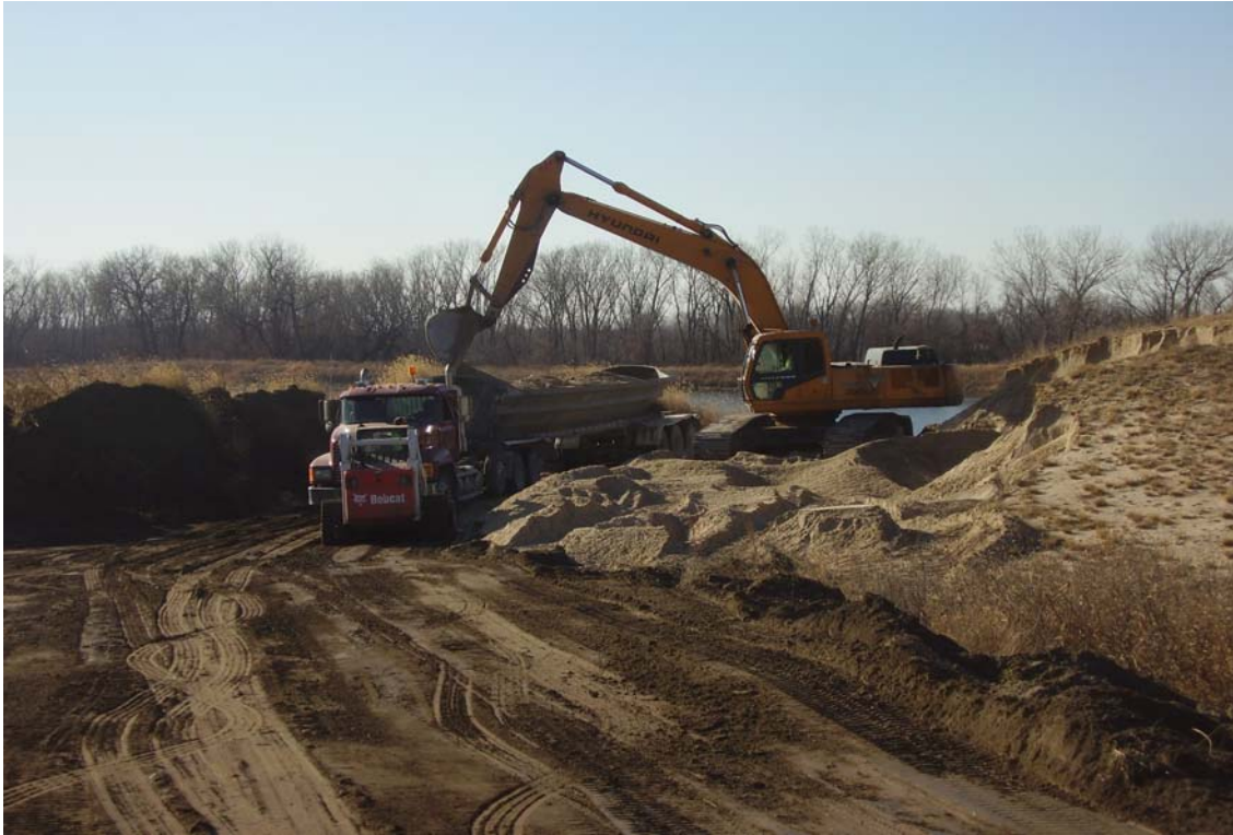
Photo: The Contractor has started hauling sand from the Jansen sandpit. Date: November 26, 2007
