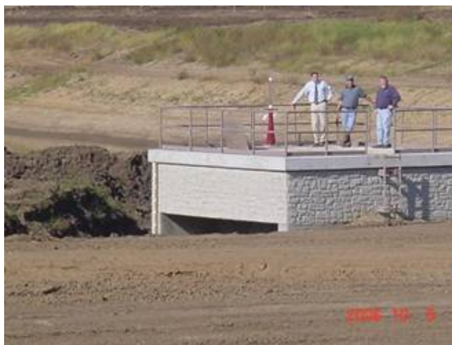
HDR Construction Oversight Engineer John Engel, NRCS Field Engineer Chuck Leinen and NRCS CET Mitch Keebler standing on the concrete box inlet for Midlands Lake. The
